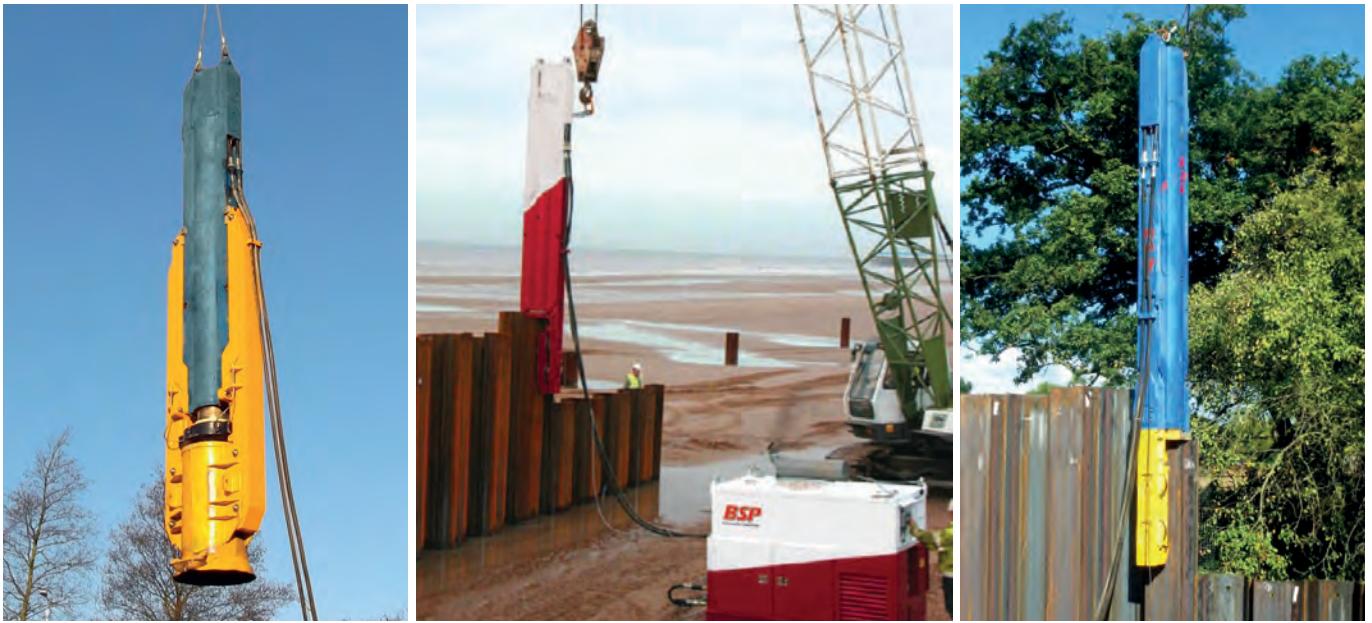
ABOVE: VARIOUS SL30 HAMMERS FITTED WITH LEGS AND INSERTS FOR DRIVING SHEET PILES. ALL ARE SHOWN IN CRANE SUSPENDED OPERATION AND POWERED BY BSP POWER PACKS.
