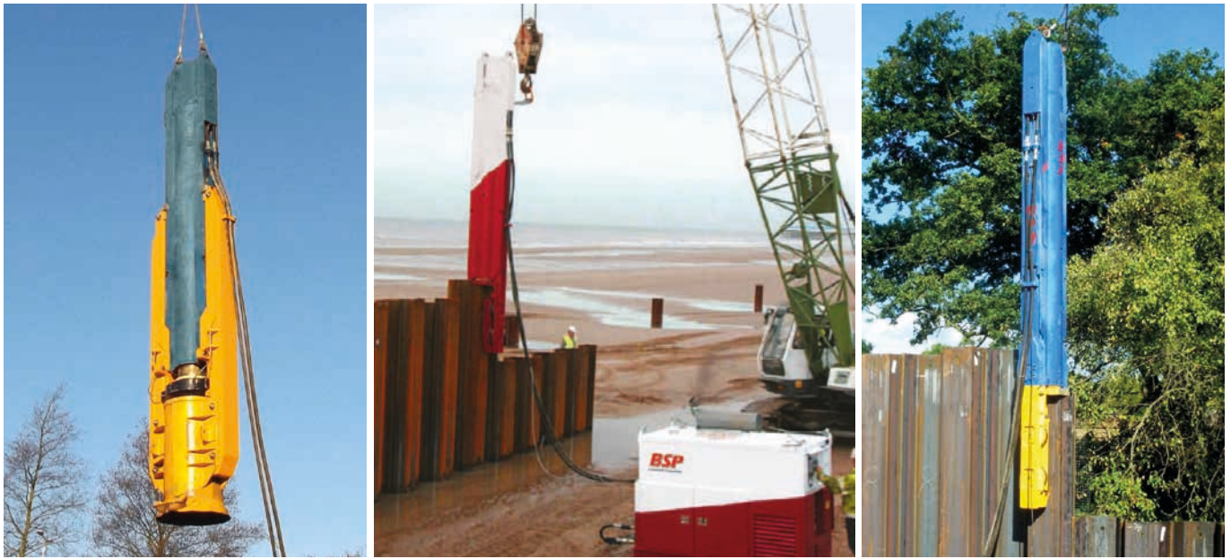
ABOVE: VARIOUS SL30 HAMMERS FITTED WITH LEGS AND INSERTS FOR DIVING SHEET PILES. ALL ARE SHOWN IN CRANE SUSPENDED OPERATION AND POWERED BY BSP POWER PACKS.
