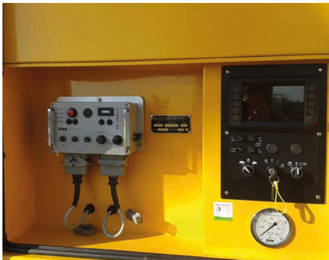
OPTIONAL CONTROL BOX MOUNTED IN HYDRO PACK
